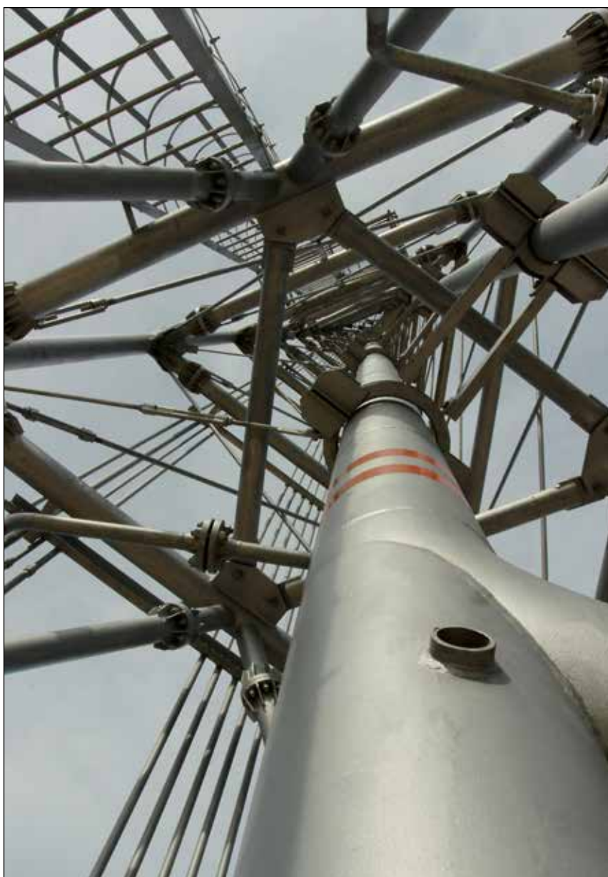
◆ Looking up the flare tower for the Songo Songo Island Gas Processing Plant
