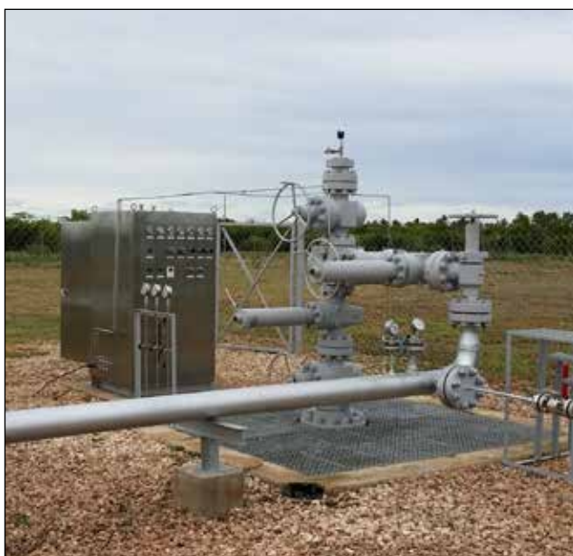
◆ Kiliwani North-1 wellhead
