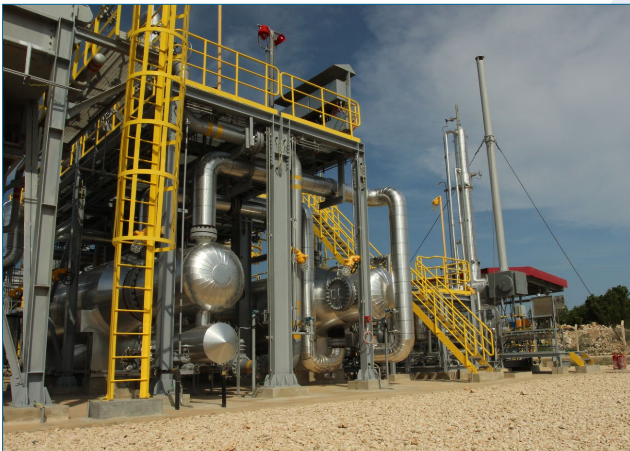
◆ Songo Songo Island Gas Processing Plant
