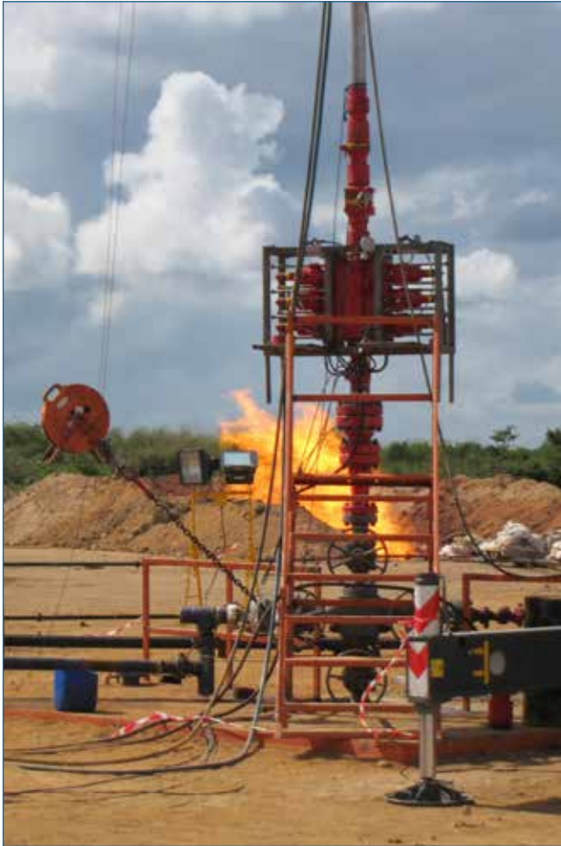
Ntorya-1 wellhead and wireline BOP with gas flare in the background
