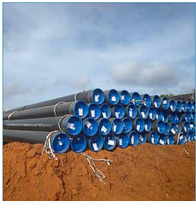
Line pipe at Ntorya to Madimba pipeline route
